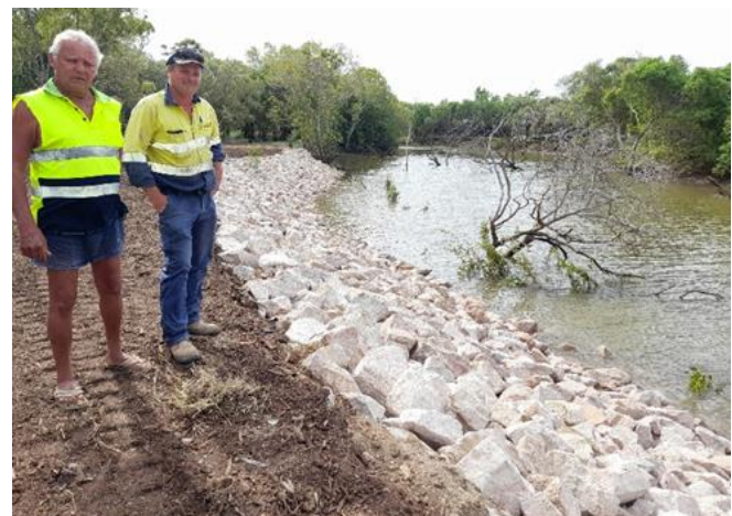
Groper Creek Caravan Park Manager Dan Garvey (left) with Olsen Contractors' Stewart Duthie
