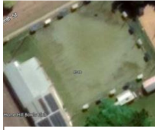
Overhead view of damage to the bowling green
