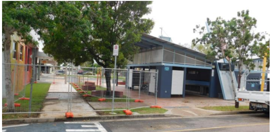
Initial work being carried out on the makeover to the Home Hill Comfort Stop by the Council
