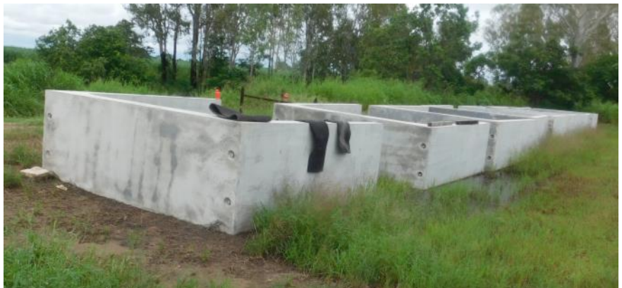
Some of the culverts being used in the construction the new bridge over Kidby's Gully
