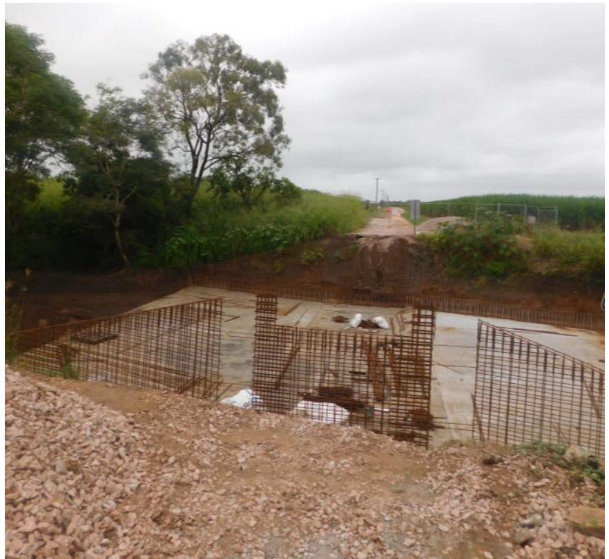
Looking down the track across the new $1 Million Haywards bridge being constructed over Kidby's Gully in the Down River section of Home Hill
