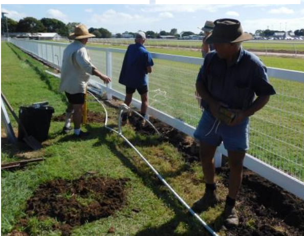
Race Club volunteers (from left) Ricky Gudge, Ron Scott, Jim Olsen (obscured) and John Woodward work on replacing the fence line between the track and the main public area
