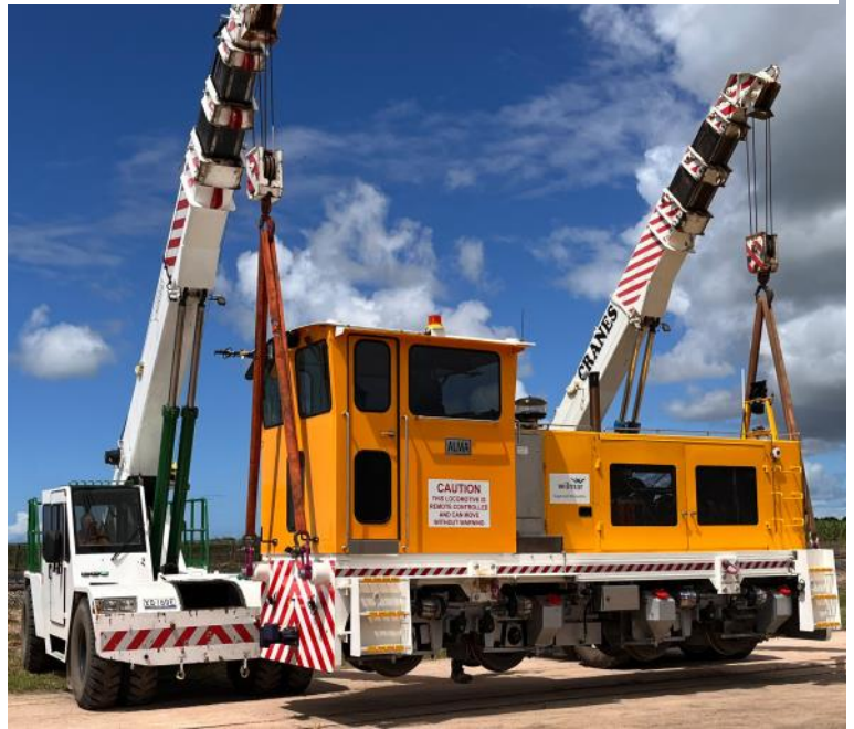
Two cranes were used to lift one of the new Inkerman Mill locos, the 'Alma' off the transport, by its front and back toe-ball, before lowering it on to the railway line .
