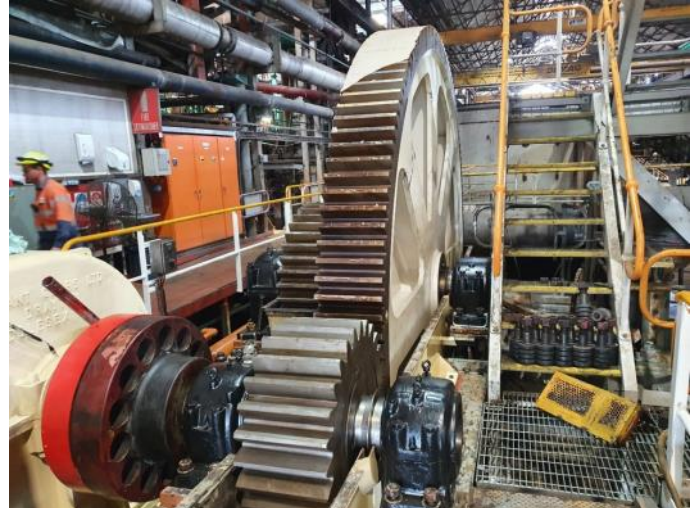
The low speed gearing on the No 1 Mill A Side at Inkerman Mill, on which work is nearing completion. (Wilmar photo supplied)
