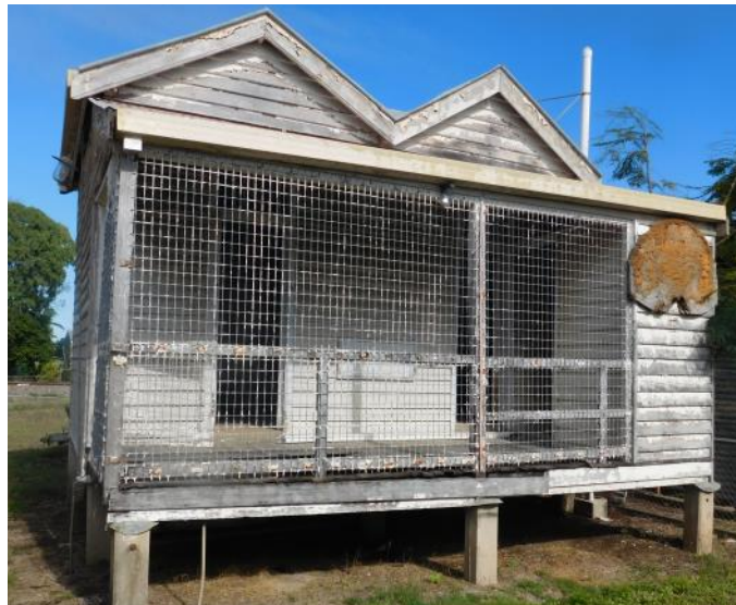
The old Watchhouse building at the back of the Home Hill Police Station, which has a long history behind its existence in the town
